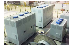
Successfully developed 10.4MVA dry type rectifier transformer
